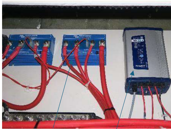
Charge distributor / shore charger
