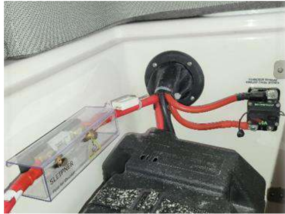
Windlass circuit breaker and fuse
