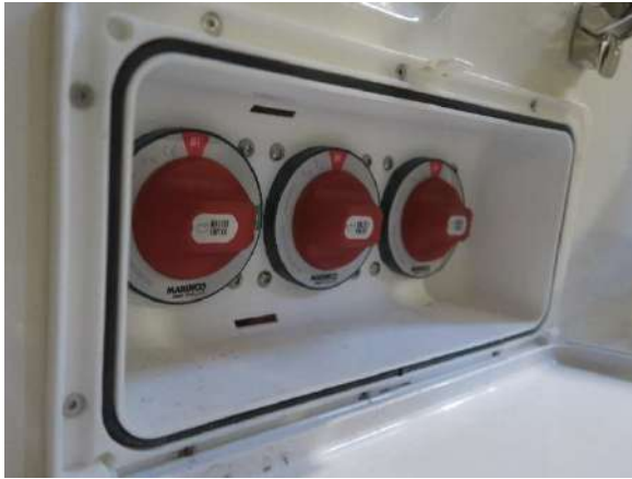
Main circuit breakers
