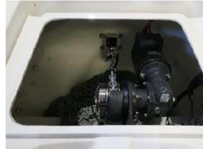
Windlass + anchor locker
