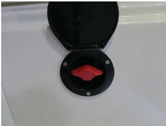
Windlass and bow thruster circuit breaker
