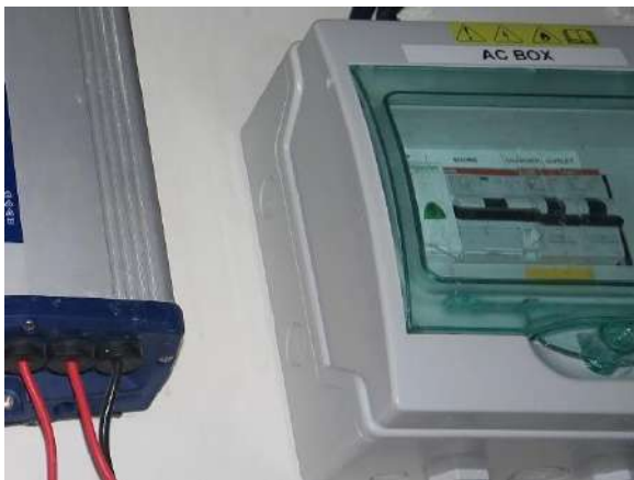
Residual current and main circuit breakers
