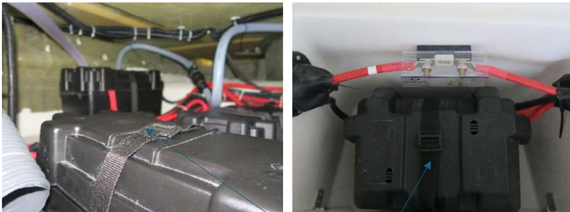
Battery detailed views (services and outboard motors / bow thruster)
